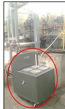
Filtration System attached to a Turbine in a Steel Plant
