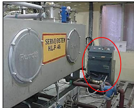
Filtration System attached to a Power Pack for critical Servo Valve
