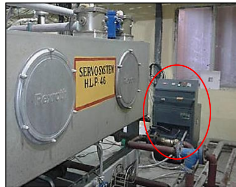
Filtration System attached to a Power Pack for critical Servo Valve
